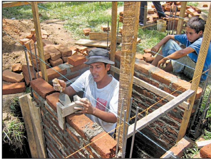
A local mason improves his masonry skills in sanitation at a training in the Matagalpa region
